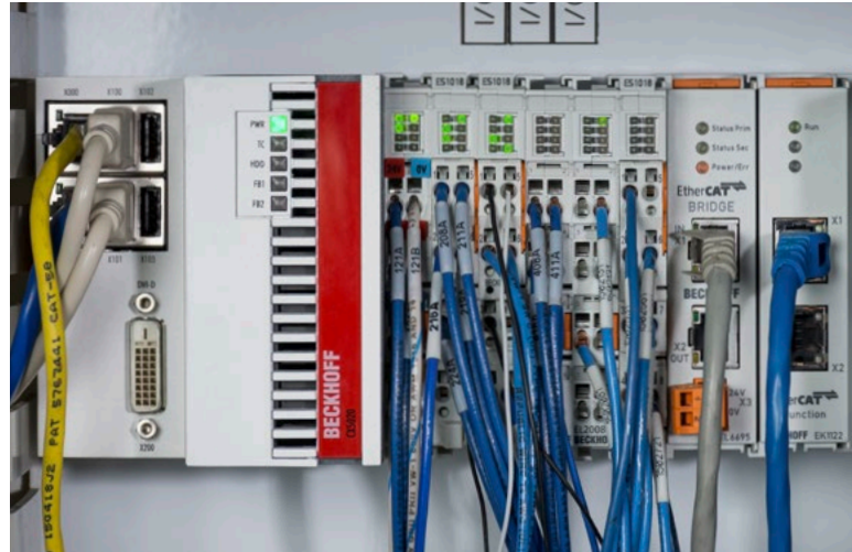
Using scalable Beckhoff Embedded PCs and EtherCAT I/O for the MC4 controls platform provided performance advantages and cost savings.
