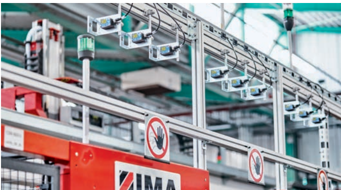
The analog signals from a total of 36 transit time sensors are acquired via the TwinSAFE SC terminals.
