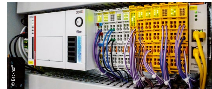
The CX2043 Embedded PC and, directly adjacent, a 130W CX2100-0014 power supply and EtherCAT and TwinSAFE Terminals provide the control hardware for this MIRACLE II project.
