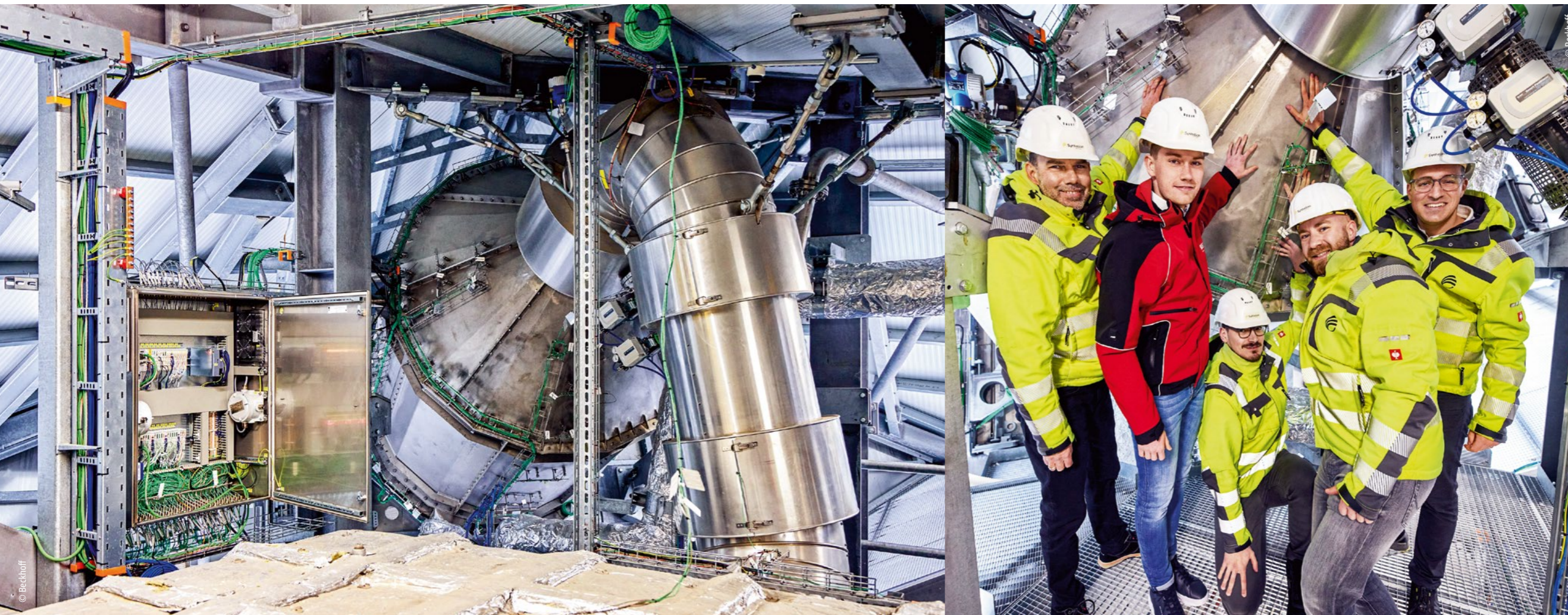
Left: The receiver with 600 kW thermal output and the ceramic energy storage unit (in the foreground) are monitored via numerous thermocouples.
