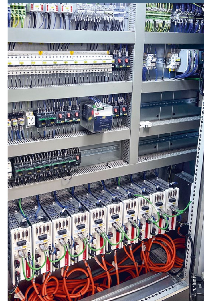
Control cabinet with numerous Beckhoff AX5000 servo drives (below)
