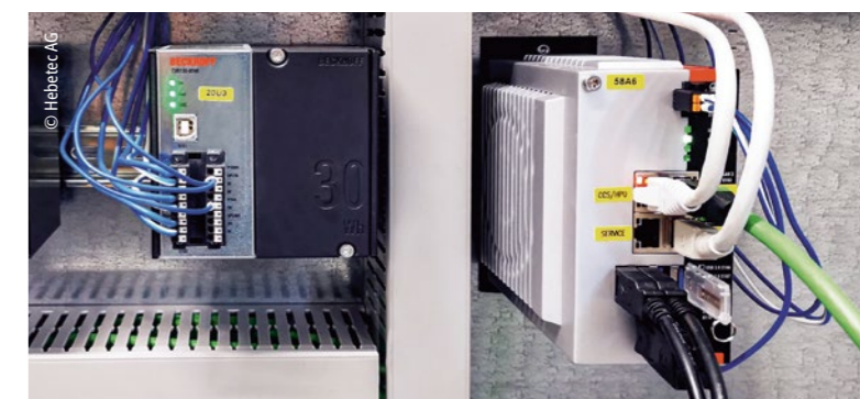
TwinCAT and C6030 ultra-compact Industrial PCs are used to control the many presses for precise leveling, uniform feed, and exact alignment of the tunnel elements.
