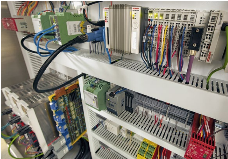
Today PakTech has an extra 20 % of free control cabinet space to accommodate additional hardware requests from customers.
